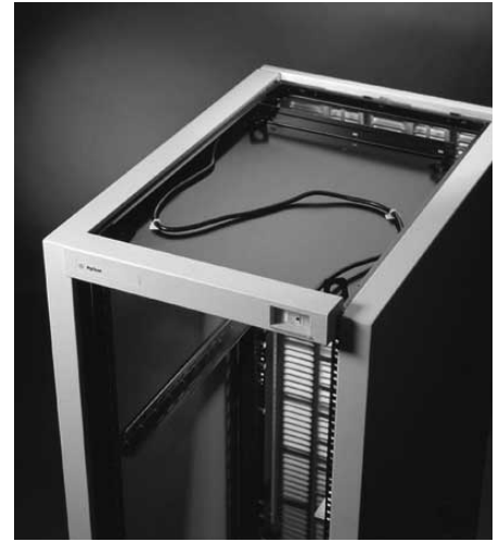
Rack with PDU and switch
